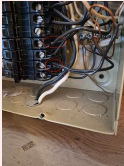
double tapped hot wires
