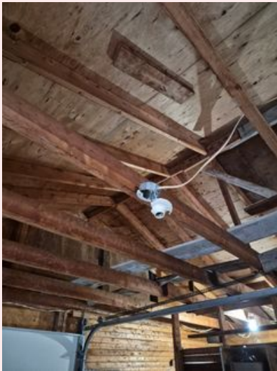
damaged light with live electrical
