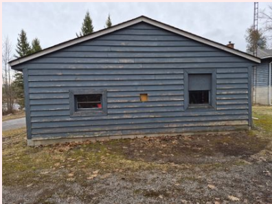
Opening in siding, rotted siding
