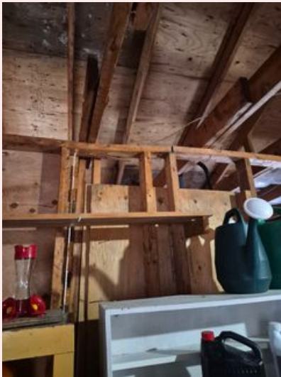
roof joists bearing weight on non structural wall
