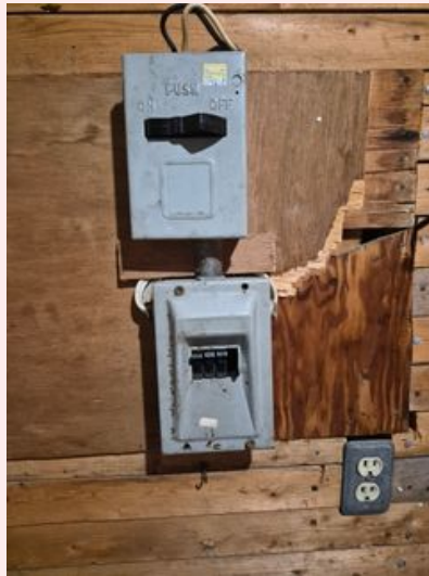
Wrong screw type in subpanel, missing screws, missing breaker plates, unprotected cables in vulnerable area, poor mounting surface.
