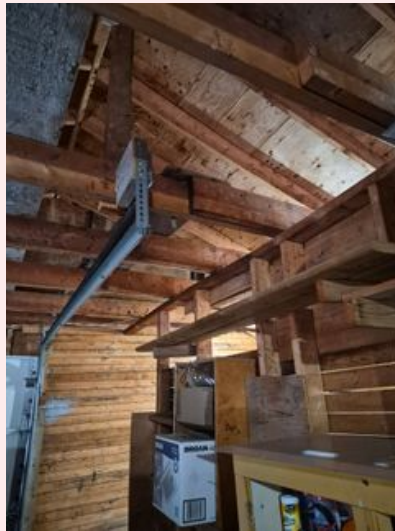
poor garage door support (2)
