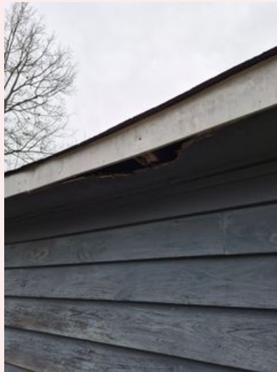
large opening in damaged soffit
