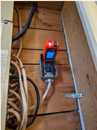
Receptacle next to electrical panel
