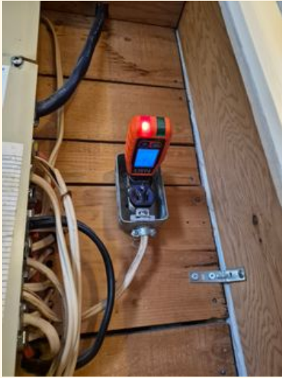
Receptacle next to electrical panel
