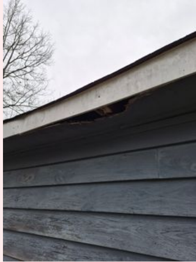
large opening in damaged soffit
