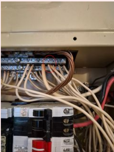
double tapped neutral wires
