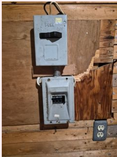
Wrong screw type in subpanel, missing screws, missing breaker plates, unprotected cables in vulnerable area, poor mounting surface.
