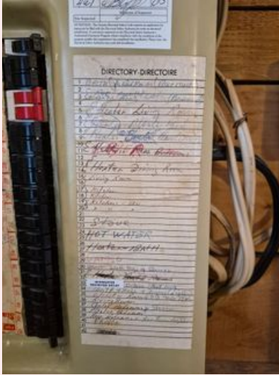
Poorly labelled panel
