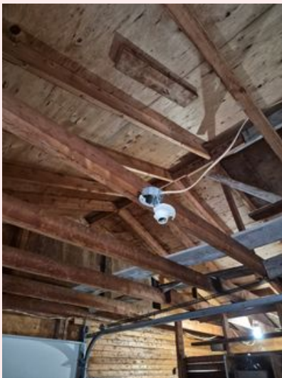
damaged light with live electrical
