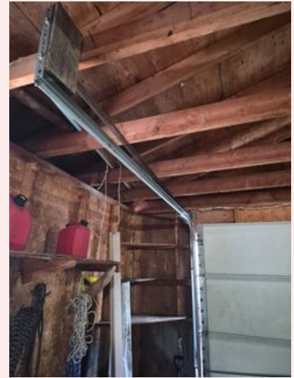
poor garage door support
