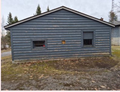
Opening in siding, rotted siding
