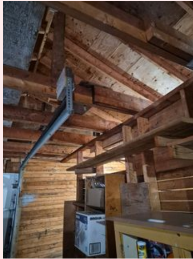
poor garage door support (2)
