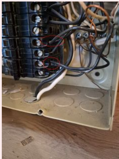
double tapped hot wires
